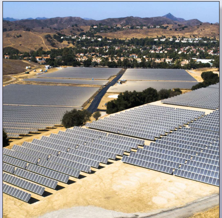
Five megawatt solar power facility used to offset the energy used by the Tapia Water Reclamation Facility
